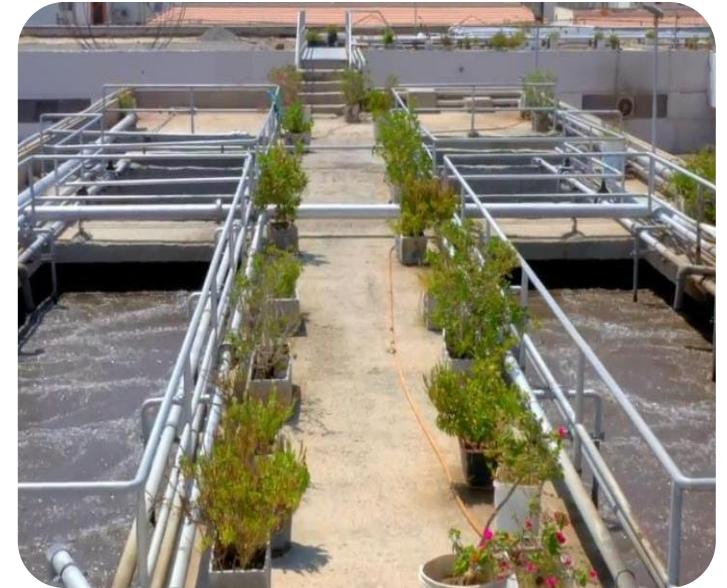
Figure: On-site wastewater treatment plant. Treated effluent feeds directly to the resort's irrigation system, closing the water loop and reducing demand on the desalination plant. Compliance with Egyptian national reuse criteria is maintained throughout the year
